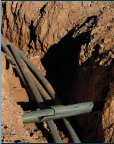
Conduit is Damaged
